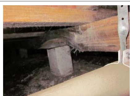
BEARER ROTTED & SLIPPING
