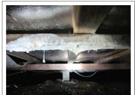
STYRENE/FOIL BETWEEN JOISTS & FUNGAL GROWTH ON BEARER
