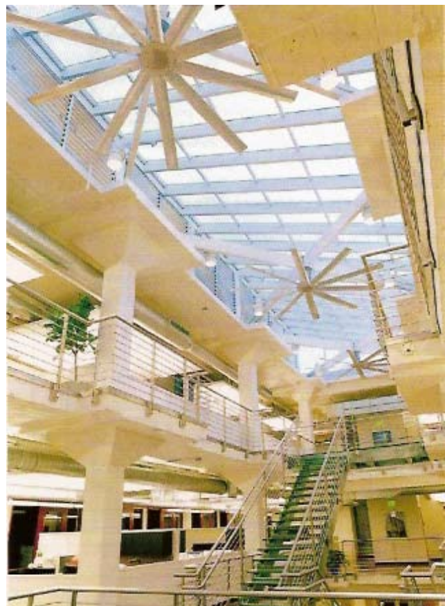
Figure 10 – de-stratification fans in air conditioned atria space
